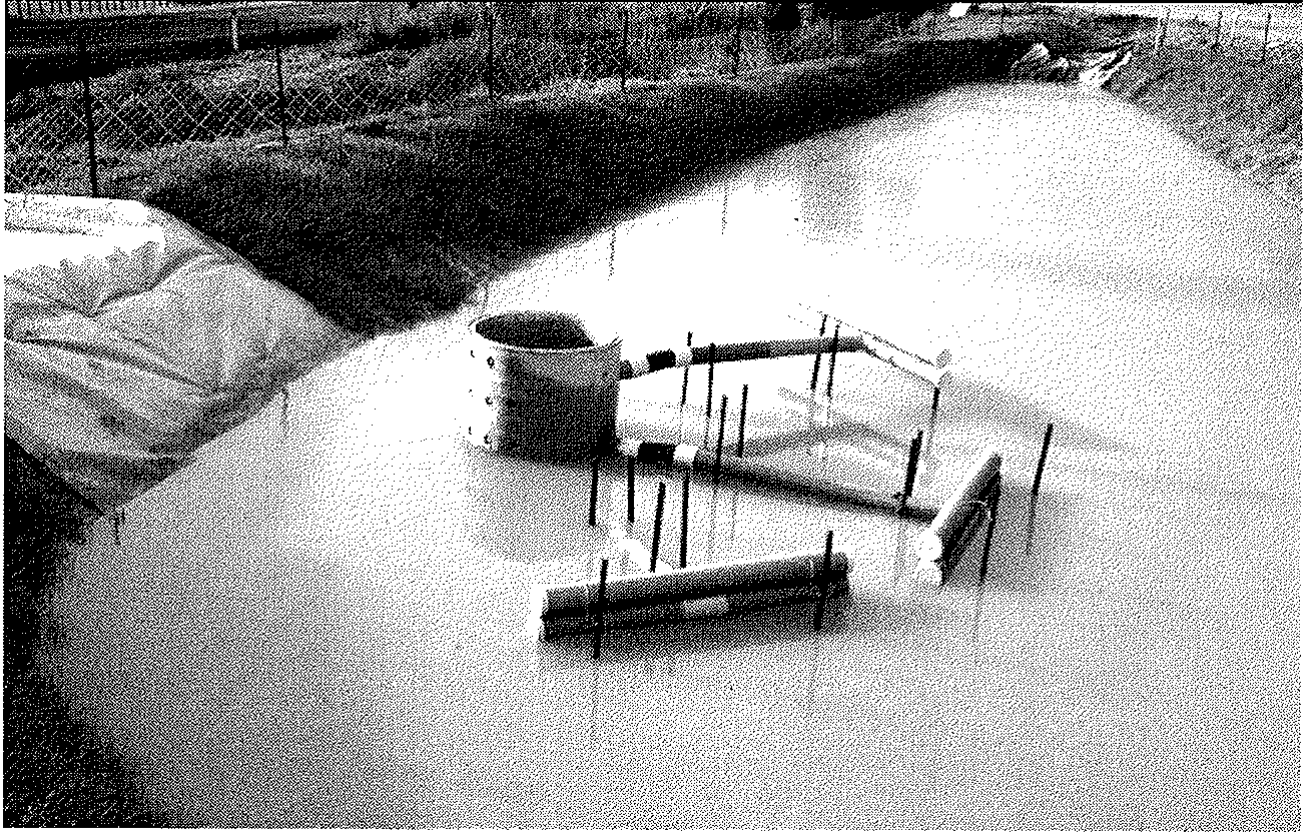
Plate 2.1.1 Sediment Retention Pond Showing Decant Systems
