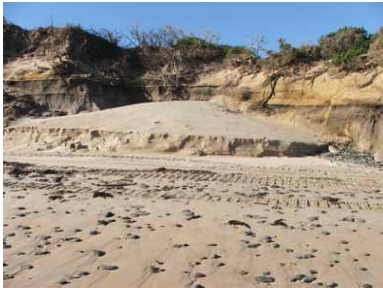
Figure 7. Collapsing unconsolidated dune sand
