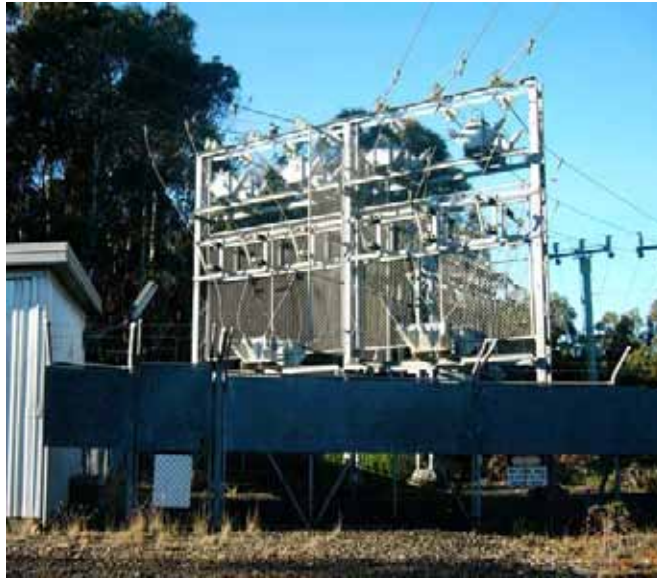
Photo 5.3.2: Electrical substation near access road to site
