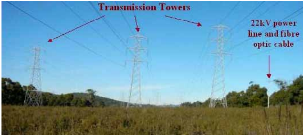
Photo 5.1.1: Power transmission corridor – looking south-east
