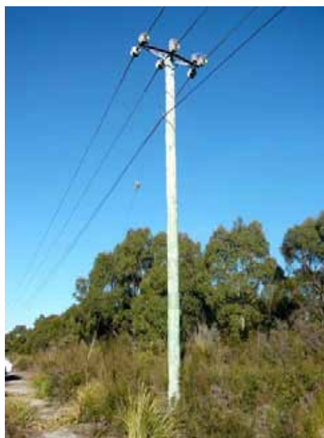
Photo 5.1.2: Existing 22kV power pole with fibre optic cable attached beneath the power lines
